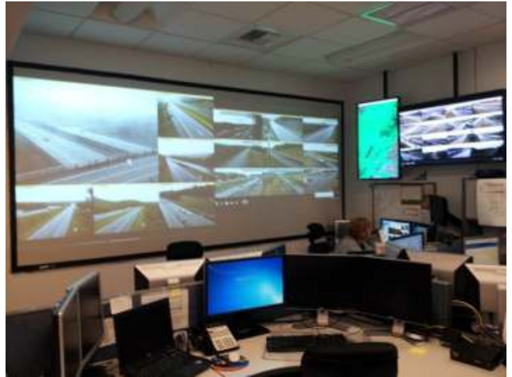
Electronics at the VDOT Traffic Operations Center in Staunton include wall and desk mounted projections of traffic conditions on I-64 at Rockfish Gap and other roads in the Shenandoah Valley.
